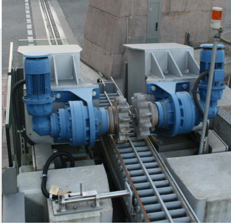
Flood protection in Hamburg’s warehouse district (Speicherstadt): in the event of a storm surge, the motorized sliding gates at Kornhausbrücke can be closed.
